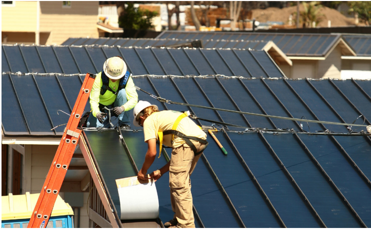
Army Hawaii Family Housing LLC (2 MW) • Schofield Barracks, Oahu, Hawaii Actus Lend Lease
